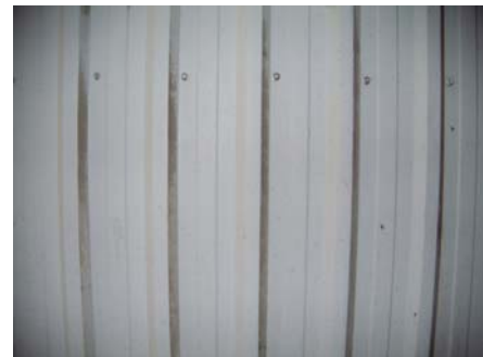
Garage Wall - Exhaust Soot - After
